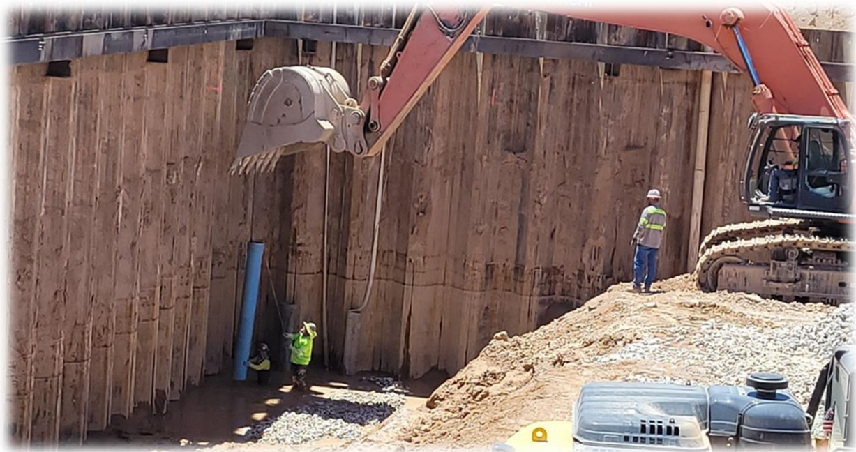
An updated dewatering system will be installed to further maximize the effectiveness of CCWRD's treatment processes.
