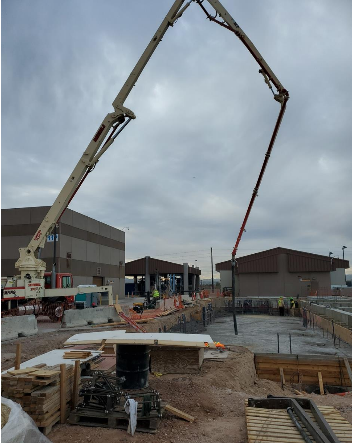
Concrete is pumped into the foundation of a new treatment facility at the Flamingo Water Resource Center
