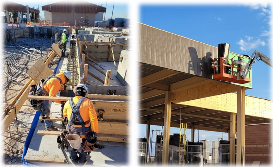
New buildings take shape on the campus of the Flamingo Water Resource Center
