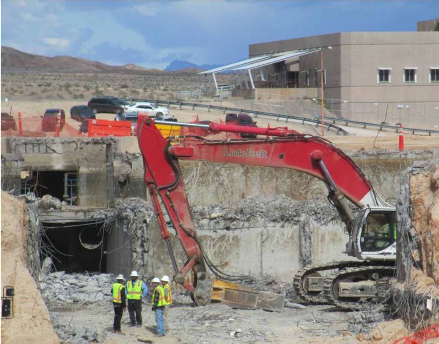
The decades-old utility tunnels were demolished as part of the East Campus demolition project
