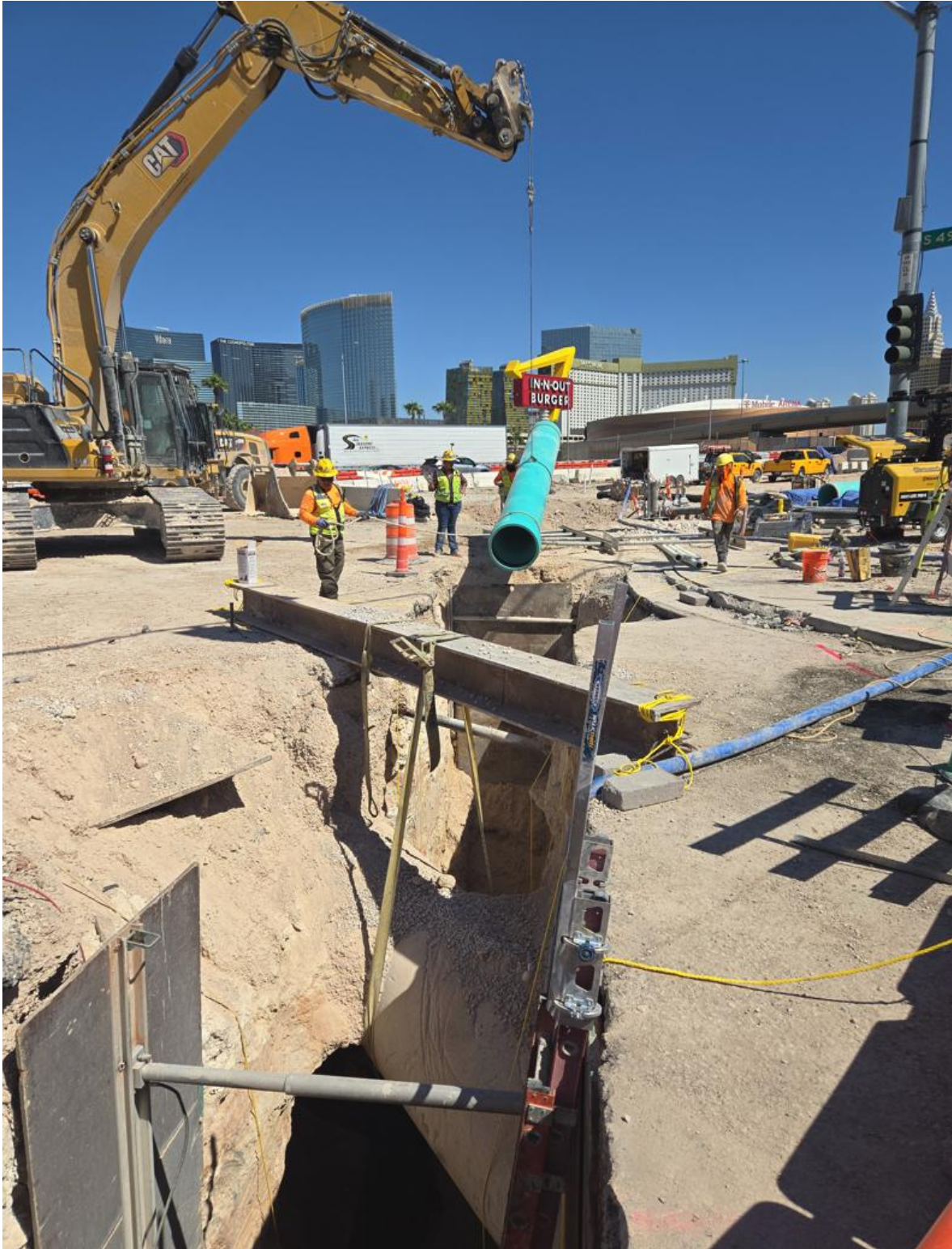
Installation of 21-in C900 PVC pipe at the NDOT Tropicana Avenue interchange project
