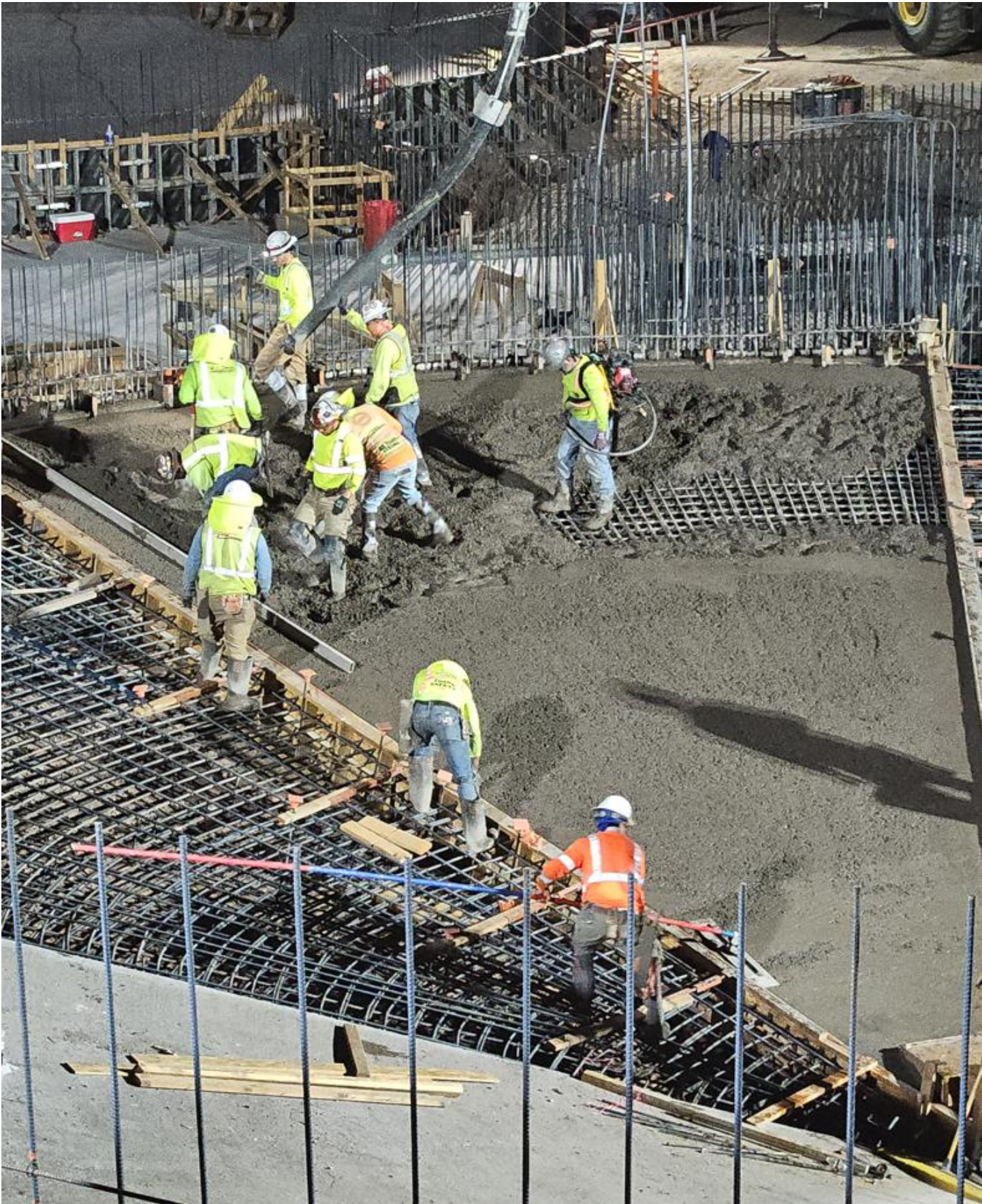
Early morning concrete pours ensure better quality concrete and protect the construction staff from the summer heat
